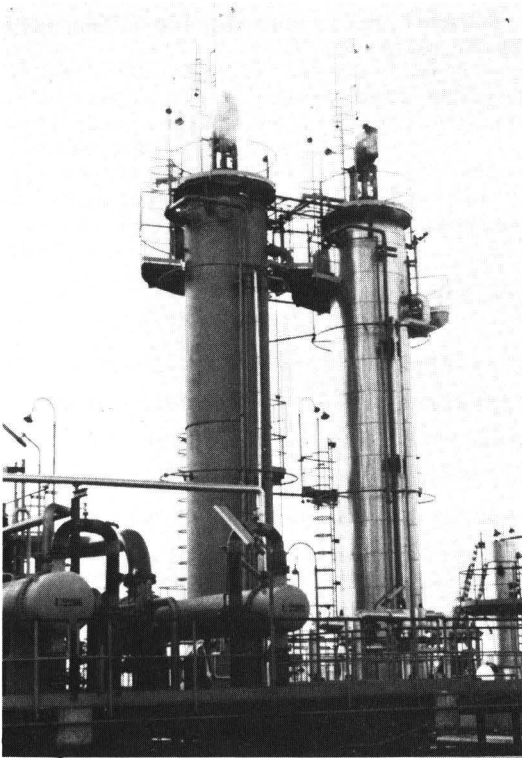
Fig. 6 Installed extraction and re-extraction column (Enichem Anic)
